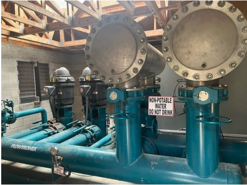
Irrigation - Pump House (Internal)
