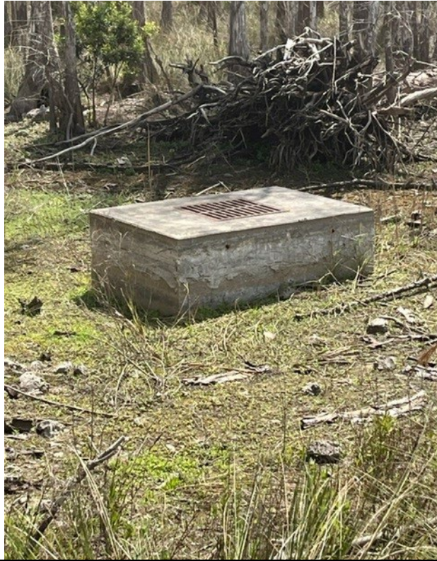
SWM – Bubble-Up Structure
